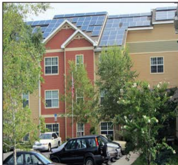
Compass Solar Energy designed and installed a 29.6 kW solar PV system to offset electric usage of the common areas of Morris Court III, a senior living community in Pensacola.
